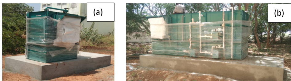
Fig-1 : (a) 5 KLD STP plant near jasmine ladies hostel (b) 20KLD STP plant back side of Science building
